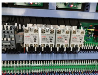
Electrical cabinet — Omron, Schneider, Fotek
