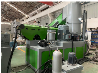
Vacuum venting system
