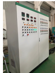
Electric control cabinet
