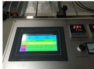
Control panel — touch screen and temperature controllers
